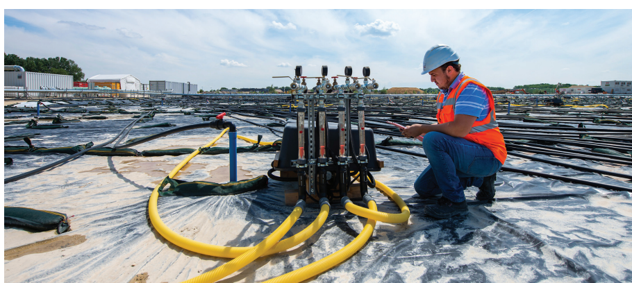
Copyright AUDI AG IN-Campus Environmental remediation of legacy refinery at Ingolstadt - air sparging unit
