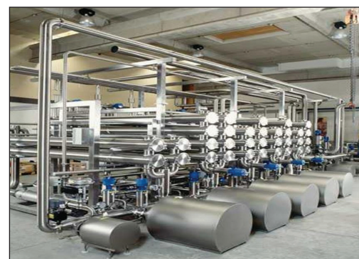
Ultrafiltration plants can turn waste products into premium products (Courtesy of GEA Process Engineering)
