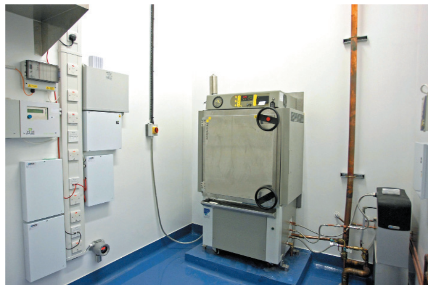
Figure 2: The service end showing the autoclave and water softener in-situ.
