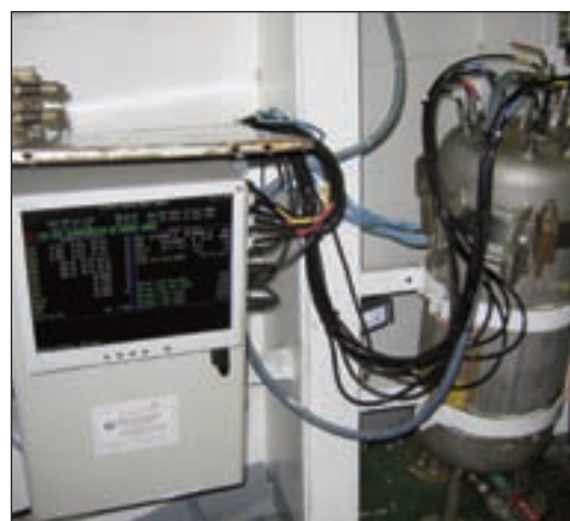
Figure 3. The SNOMS sensor tank and data logging unit in the machinery space of the MV Pacific Celebes
