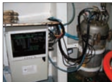
Figure 3. The SNOMS sensor tank and data logging unit in the machinery space of the MV Pacific Celebes
