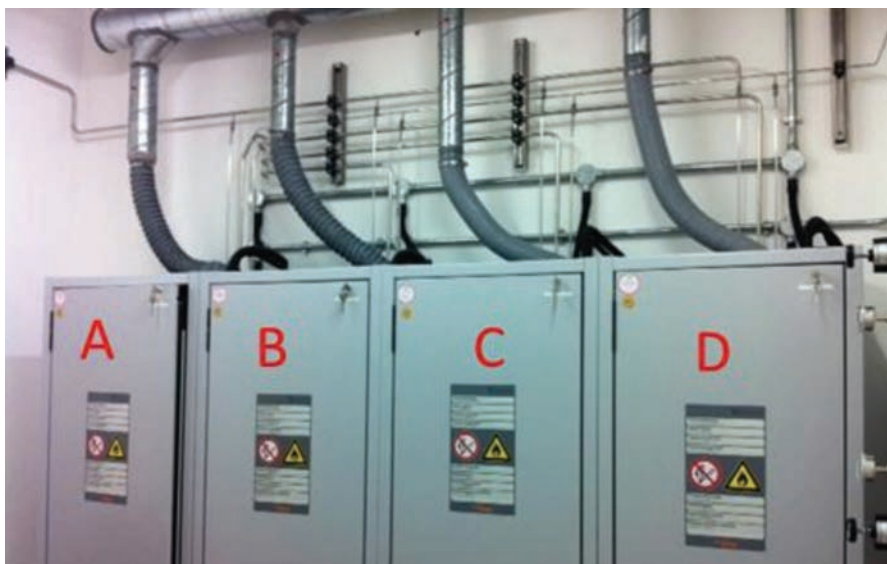
Figure 2: SFC co-solvent delivery room and flammable solvent cabinets for each solvent type methanol (A), ethanol (B), isopropanol (C) and special solvent blend as required (D).
